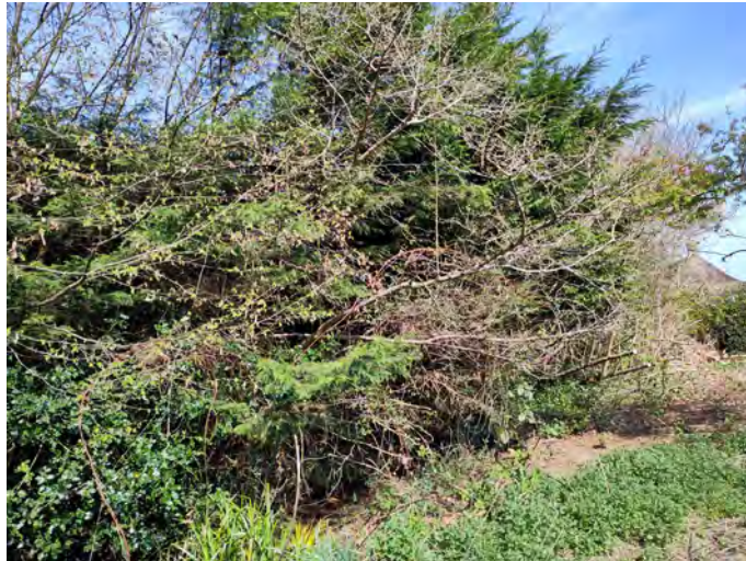
Hedge overhanging the ditch
